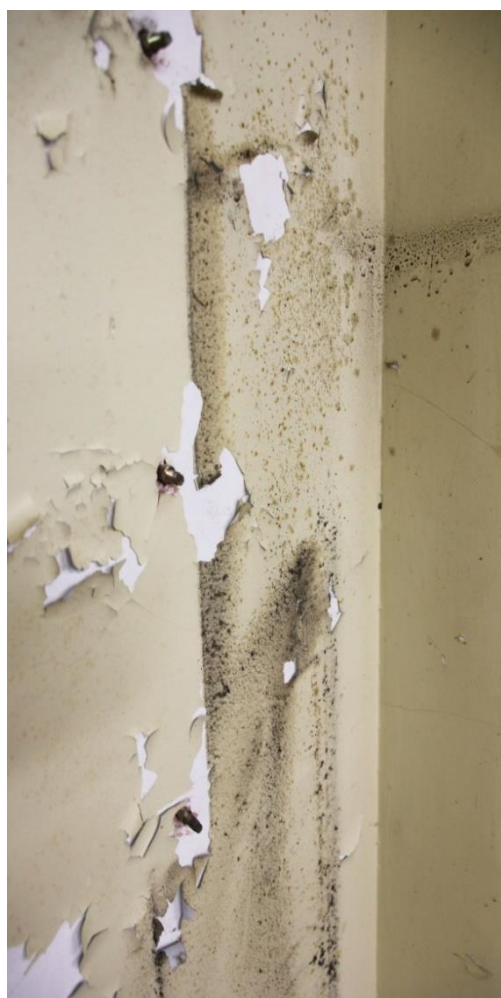
This corner harboured a dead air pocket and trapped moisture, causing black mould to form and the paint to peel.
